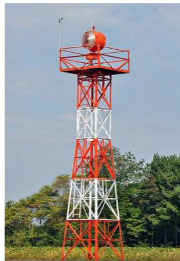
Crouse Hinds DCB-225 rotating beacon on tower
