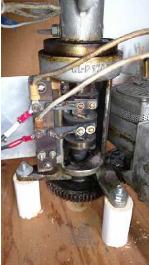
1944 vintage rotating brass slip rings and contact brushes provide 110v current to W28 beacon bulb
